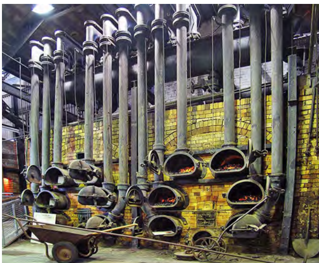
An array of retorts at the gasworks. Photo Tarboat
